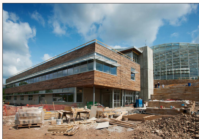
The Phipps Conservatory's Center for Sustainable Landscapes is under construction and expected to be completed this summer.
